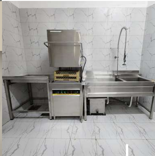
Wash Up Area Run out Table , Dish washer, Pre rise minxertap & Sink
